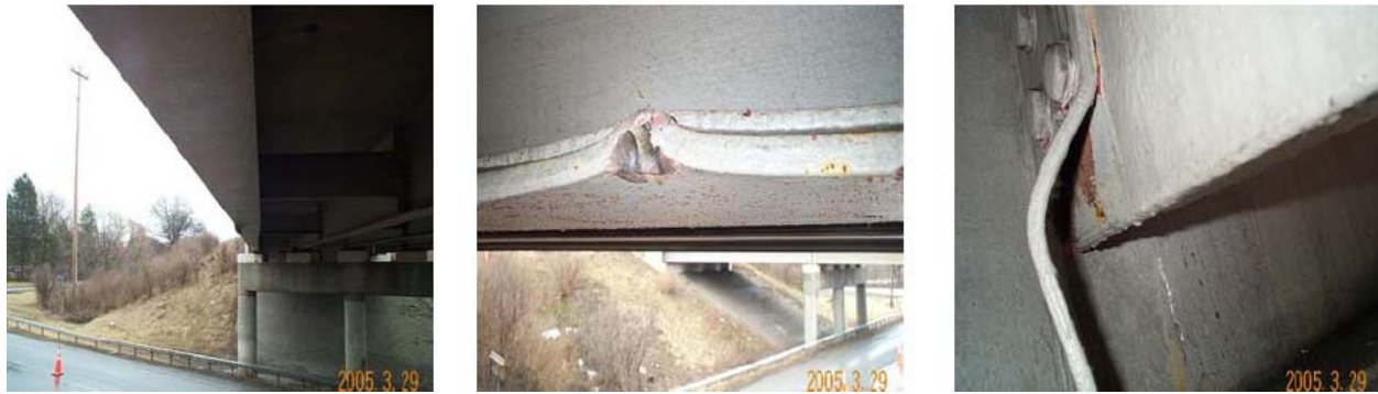
Figure 3-8: Damages to the Bridge 1062872 on the Route 400 over Jamison Road Observed During an Inspection.
