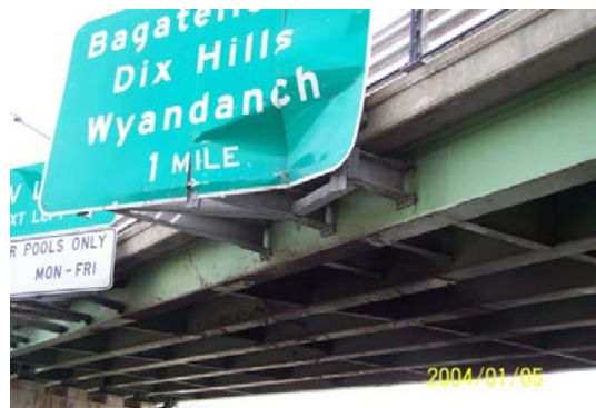
Figure 3-24: Damage to the Sign on the Bridge 1049310 Over I-495.
