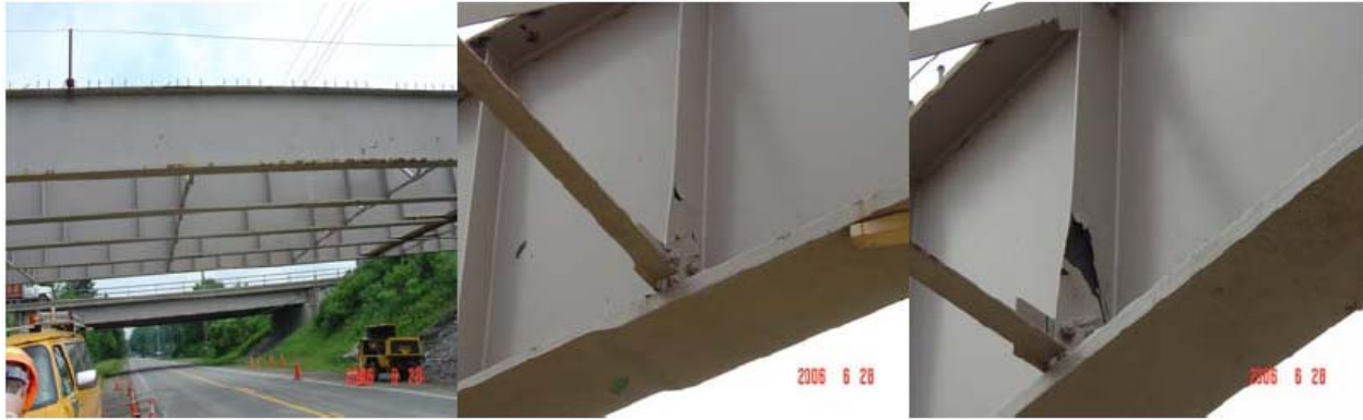
Figure 3-7: Damages to the Bridge 1092032 Observed During an Inspection.
