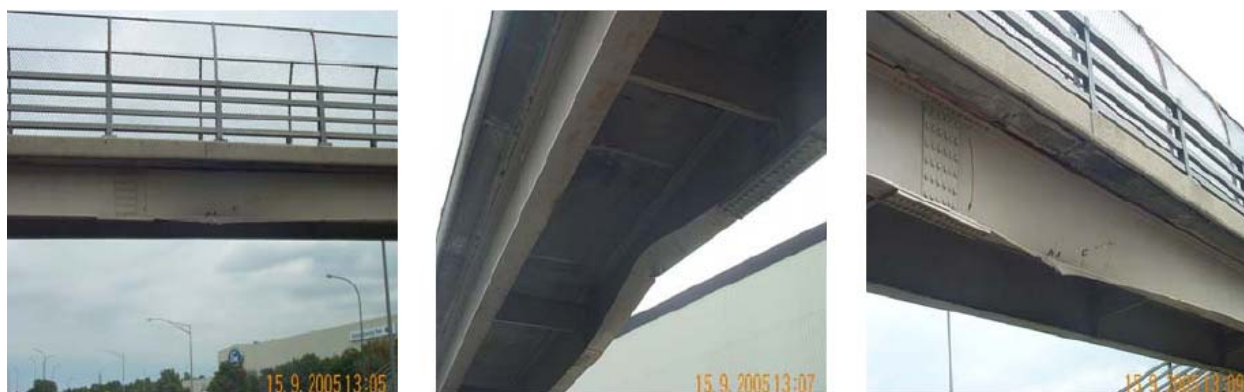
Figure 3-6: Damages to the Bridge 1001410 Observed During an Inspection.
