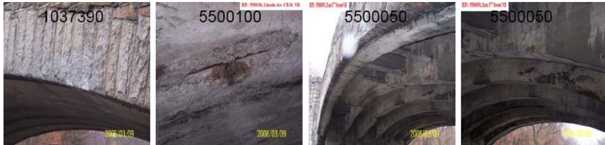
Figure 3-18: Typical Damages to the Bridges in Region 8 because of Multiple Hits.
