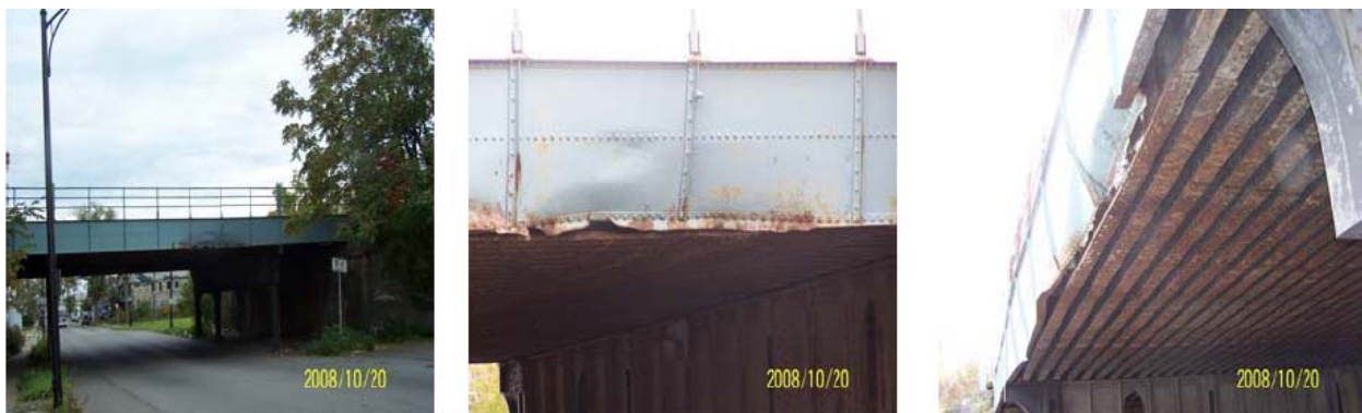
Figure 3-3: Damages to the Girder of Bridge 7708160 Because of Multiple Hits.
