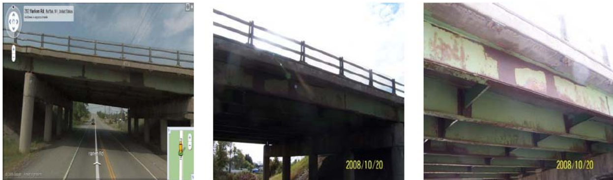
Figure 3-2: Damages to the Girder of BIN 5060589 Because of Multiple Hits.
