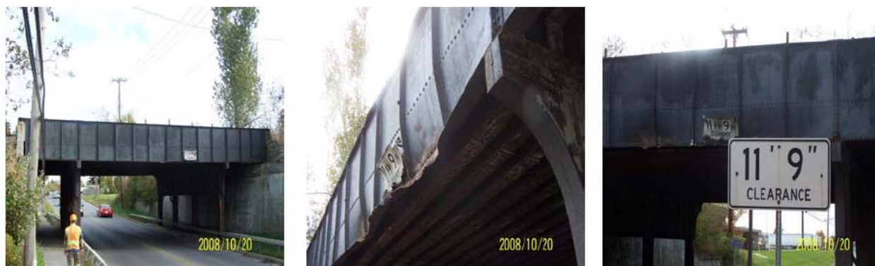
Figure 3-4: Damages to the Front Face of the Bridge 7708610 Because of Multiple Hits.
