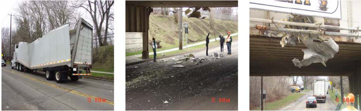
Figure 3-13: Impact to the Bridge 7707520.
