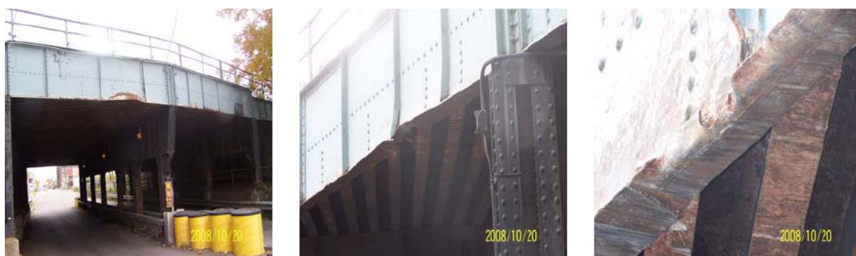
Figure 3-5: Damages to the Front Face of the Bridge 7046420 Because of Multiple Hits (hit 41 times).
