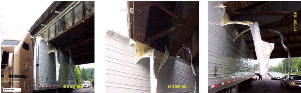
Figure 3-9: Impact to the Bridge 7050631 on Big Tree Road in Hamburg, New York.
