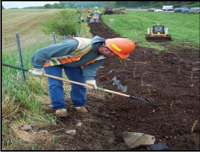
Dale Neu of Onondaga East Residency doing final work placing mulch. Mulch, placed with an excavator or shovel, is an important final step to conserve moisture and discourage weed growth.
