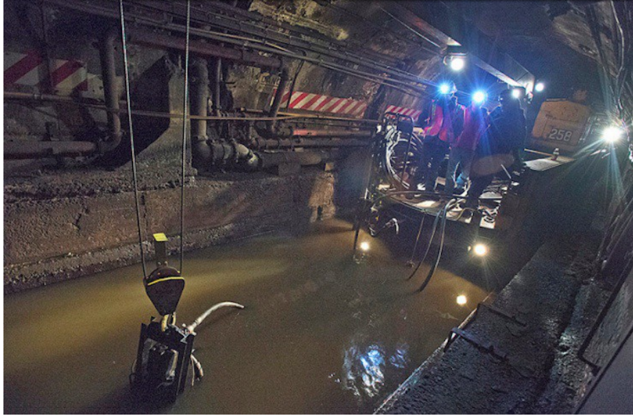
Transit workers pump seawater out of the Canarsie tunnels after Hurricane Sandy on November 5, 2012 Metropolitan Transportation Authority / Patrick Cashin
