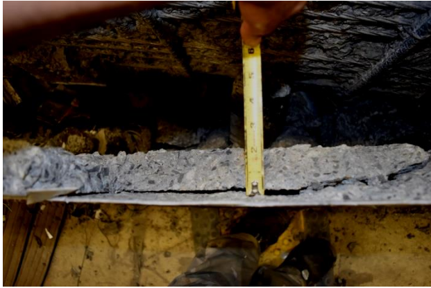
a) spalled concrete cover
