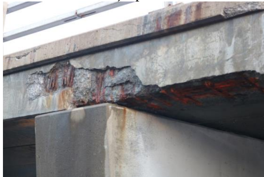
b) damage at the pier support
