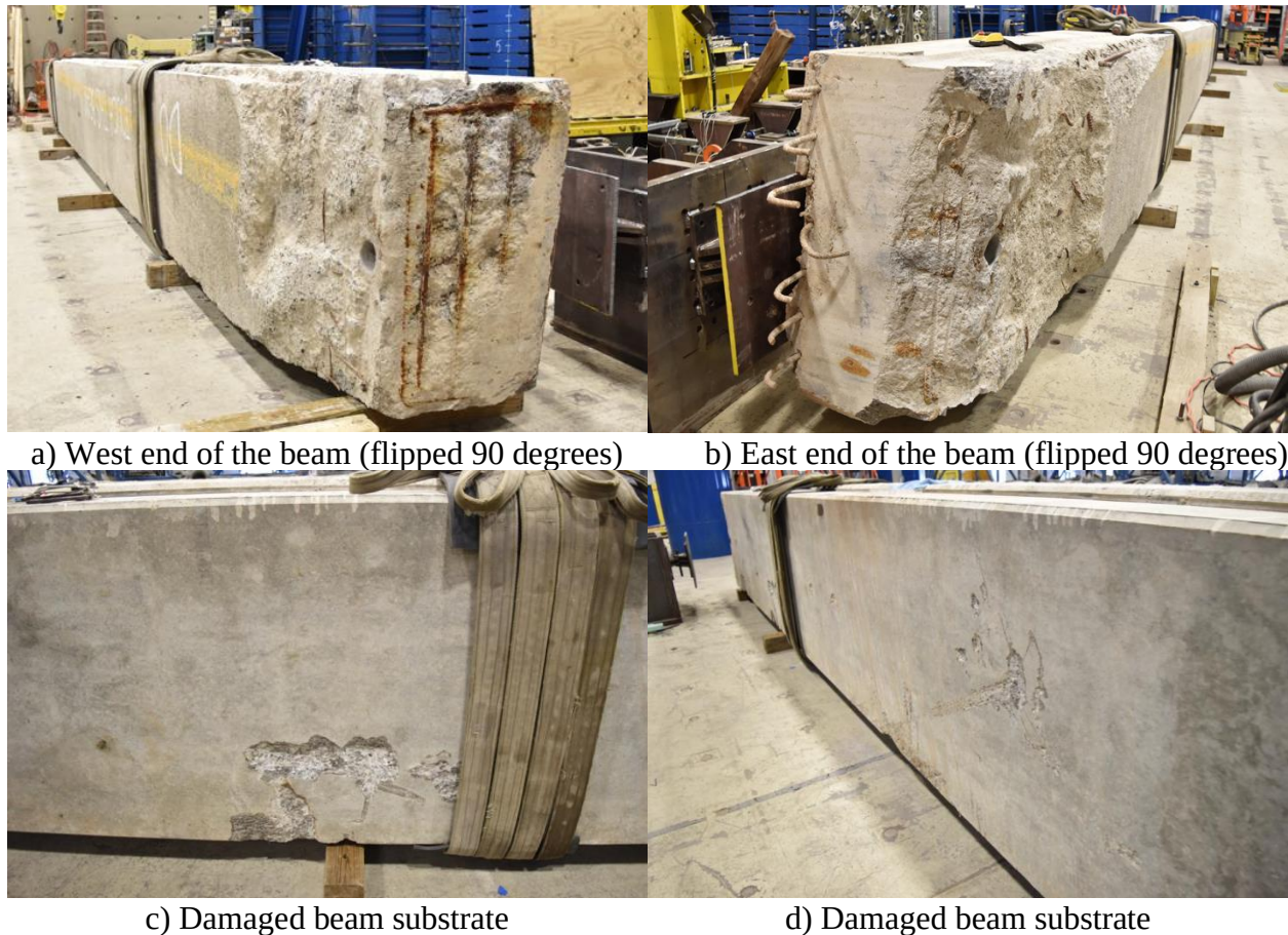
Figure 2-8 Overall condition of Beam 3 upon delivery to the SEES laboratory
